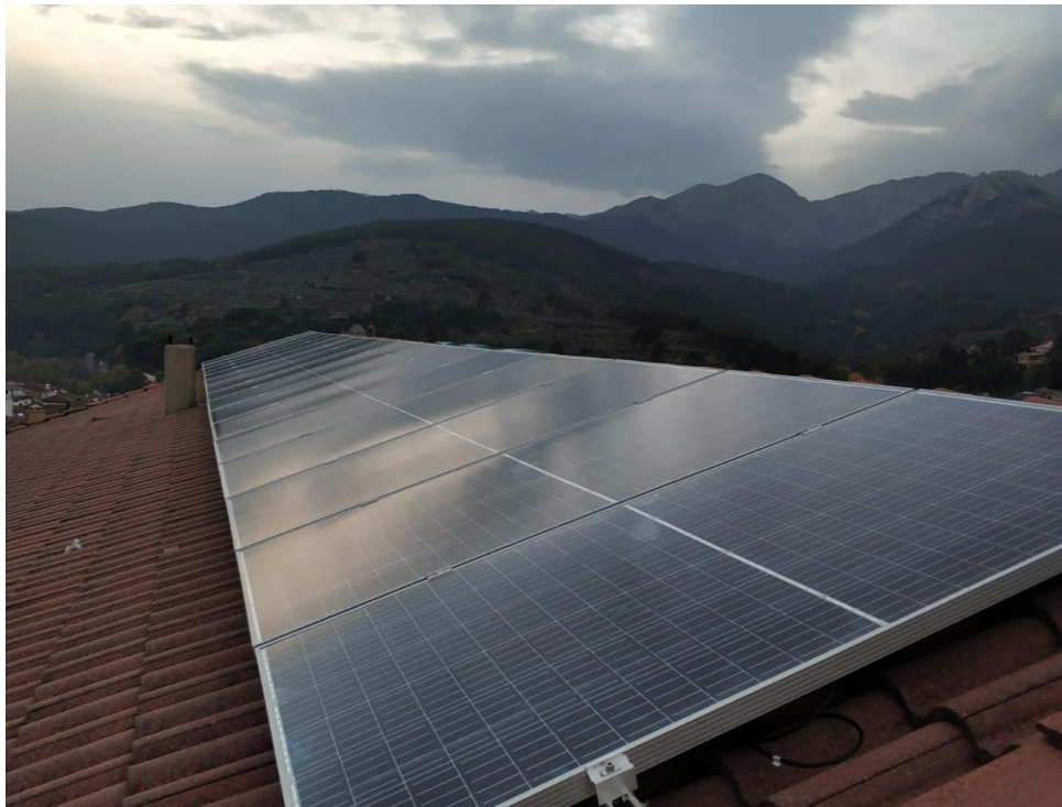
Solar panels in one of our residences (Residencia Don Bosco, Madrid).
